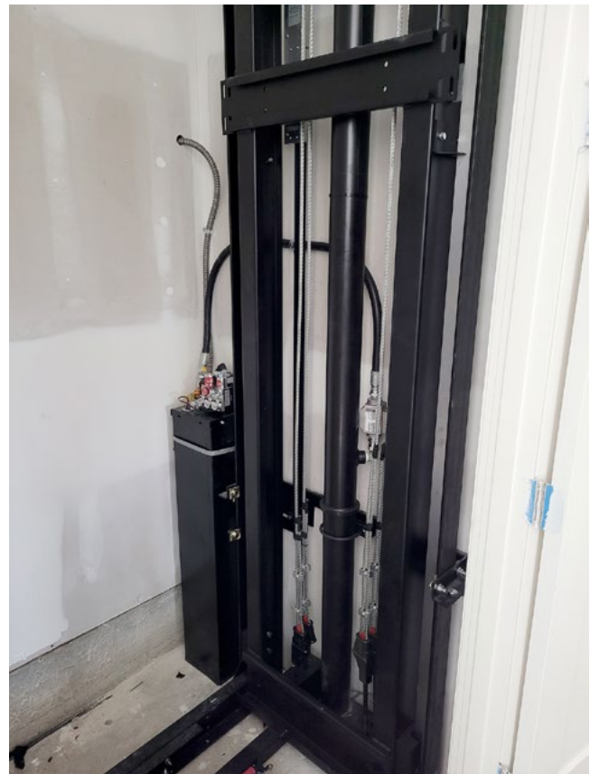
MRL pumping unit with remote controller.
